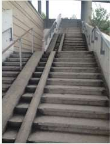
A stairwell built to accommodate both bicycles and strollers on the campus of NTNU in Trondheim, Norway.
